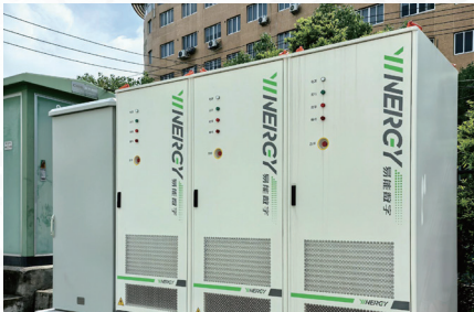
Zhejiang Jinhua General Equipment 300kW/645kWh
