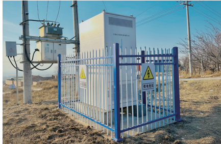
Ningxia Guyuan Rural Area Energy Storage 100kW/215kWh
