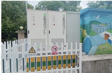
Zhejiang Taizhou Electrical Machinery 200kW/430kWh
