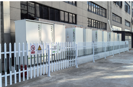
Zhejiang Taizhou Rubber & Plastic Manufacturing 800kW/1720kWh
