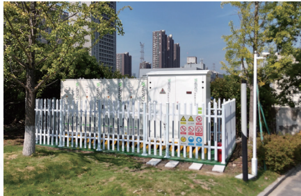
Zhejiang Hangzhou Electronic Equipment 400kW/860kWh
