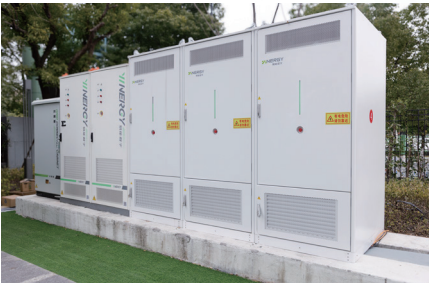
Zhejiang Hangzhou Energy Service Industry 500kW/1075kWh
