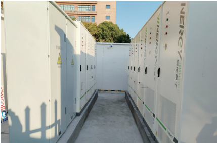
Zhejiang Hangzhou Telecom Operator 1000kW/2150kWh
