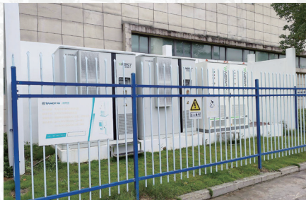
Zhejiang Wenzhou Meter Manufacturing 400kW/860kWh
